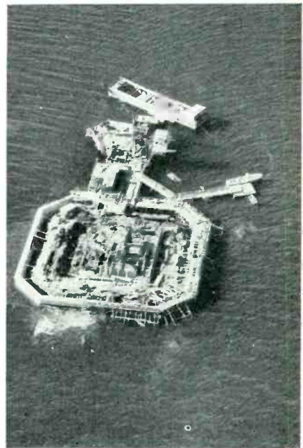
This Fairchild Aerial Survey photograph shows the construction of foundations for the new WABC station at West Pea Island in Long Island Sound
